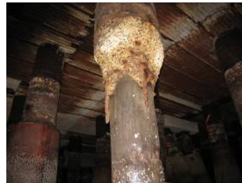
Marine infrastructure in various states of deterioration
